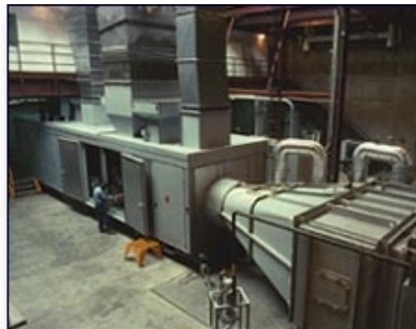
Figure 2-6. Rolls-Royce Allison 501-K Turbine Power Package
