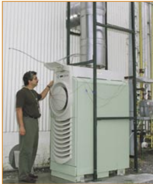
Modular microturbines are best suited for commercial and institutional applications, but can be connected together for larger industrial uses.
